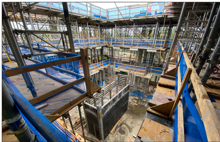
Internal view of the construction on the Judy Genshaft Honors College facilities
